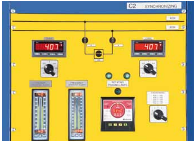
Synchronising panel of the Power Plant Module.
