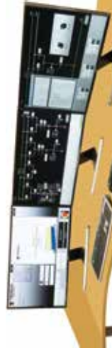
PST2250-15 SCADA System
