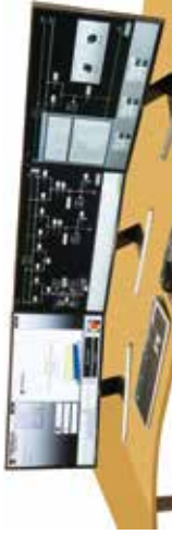
PST2250-15 SCADA System
